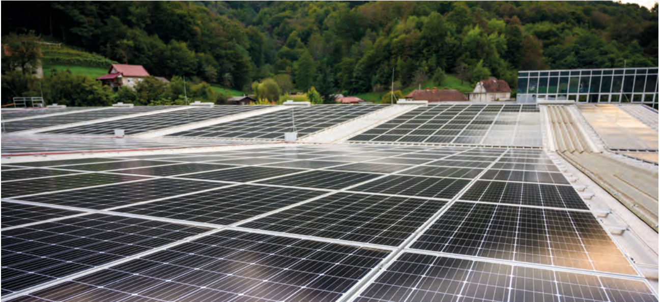
The existing 3,400 solar panels are located on the roofs of the finished goods warehouses, a previously unused area.
